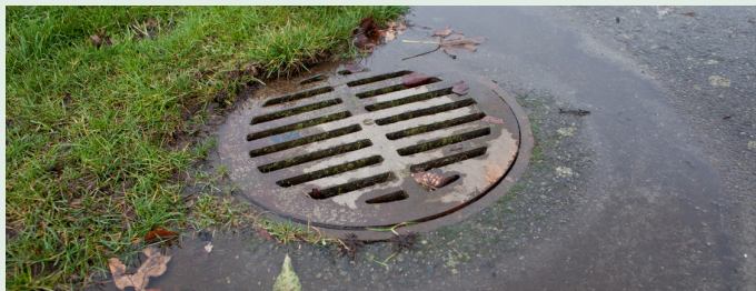
WHAT DRAINS IN HERE
